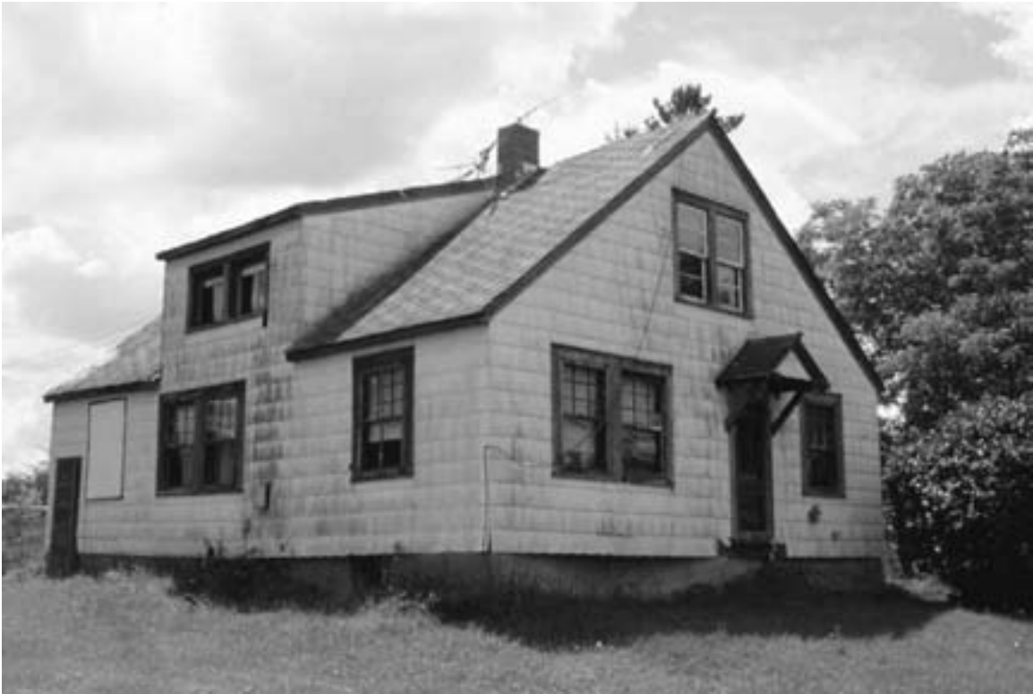
A farmhouse with asbestos-cement siding. Kathio Township, Mille Lacs County, 2003. (Gemini Research photo)
