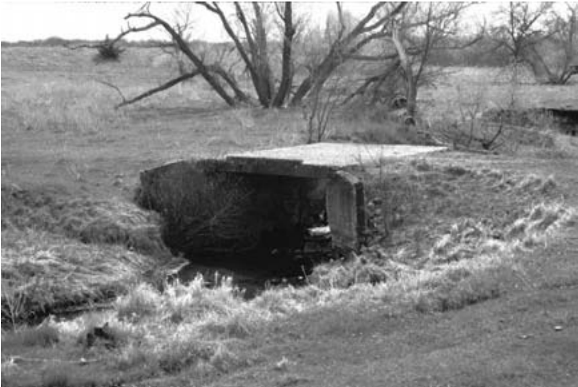
A poured concrete bridge (reinforced with iron) that carries a narrow farm lane over a stream in Stearns County. 2004. (Gemini Research photo)
