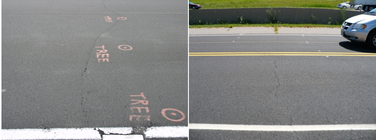
Figure 3. Typical Cracking Pattern on Cell 6 (Left) and Cell 31 (Right)
